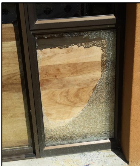
Figure 1: Broken window, allegedly by SWB6, at the Bluegums area
